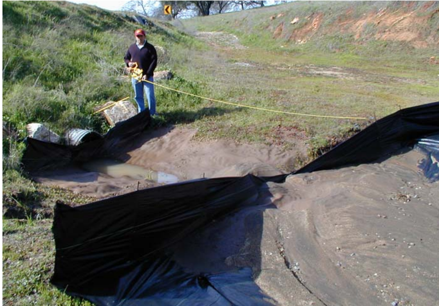
(a). Trapped sediments in Sediment Traps 1 and 2 (beside Rd 415).
