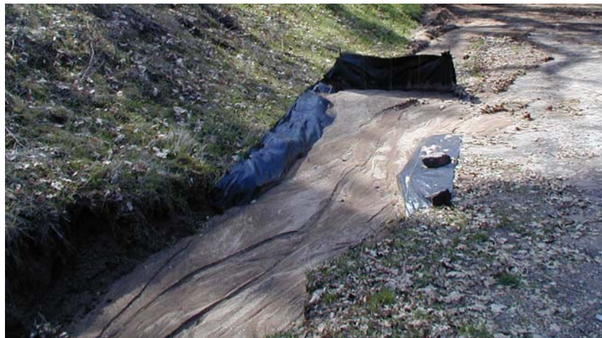
(b). Trapped sediments in Sediment Trap 3 (beside Rd 600).
